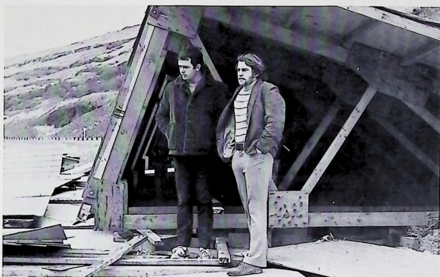
WSU Coach Robert Orr and unidentified oarsman inspect storm damage.
